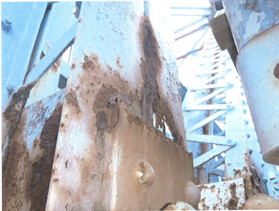
Figure 5: Photo of Recommended Repair Location at Road Bridge
