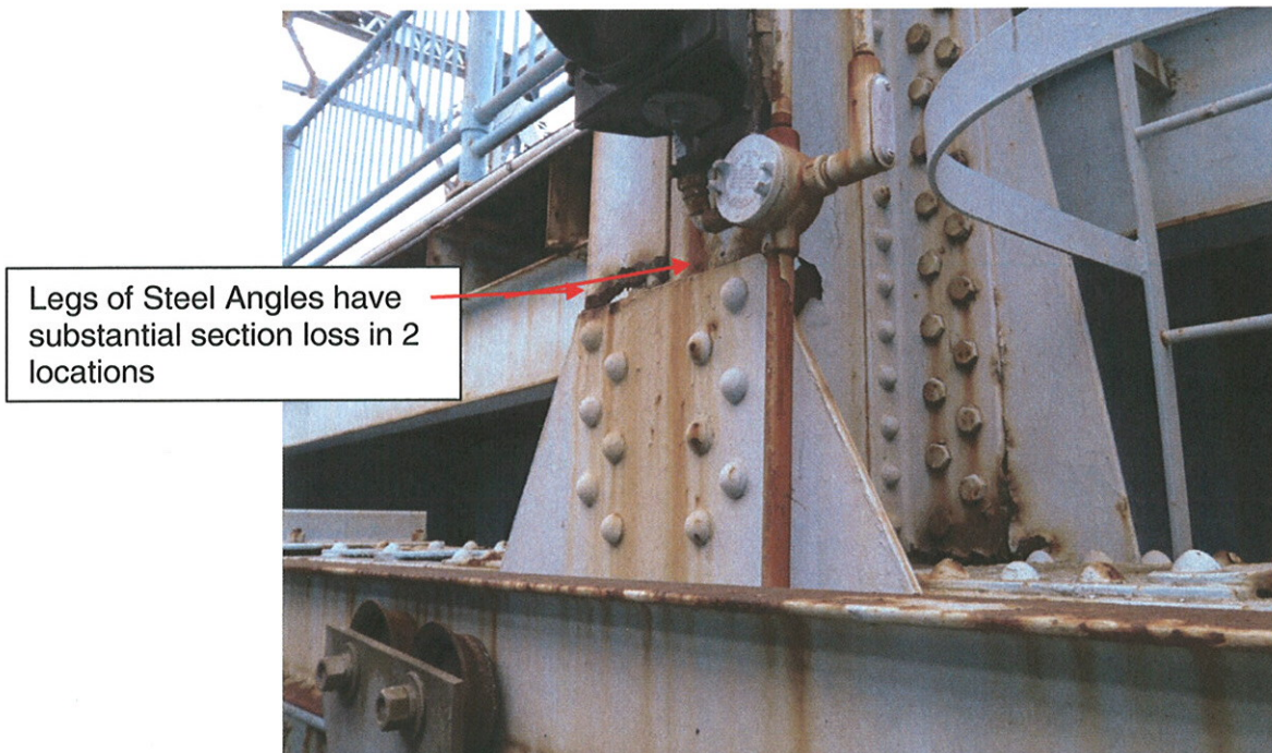
Figure 2: Photo of Critical repair 1 at Rail Bridge
