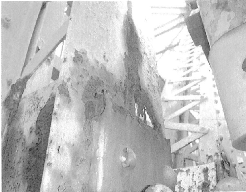
Figure 5: Photo of Recommended Repair Location at Road Bridge
