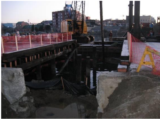
Removing a timber pile- note debris boom and silt curtain against upland bank
